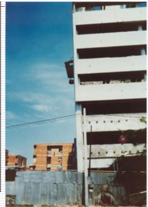
Failures of building foundation Due to excavation in Underconsolidating soils
