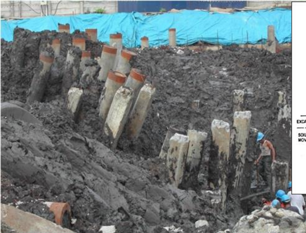
Excavation cause sliding and Tilting (and breaking) of Piles
